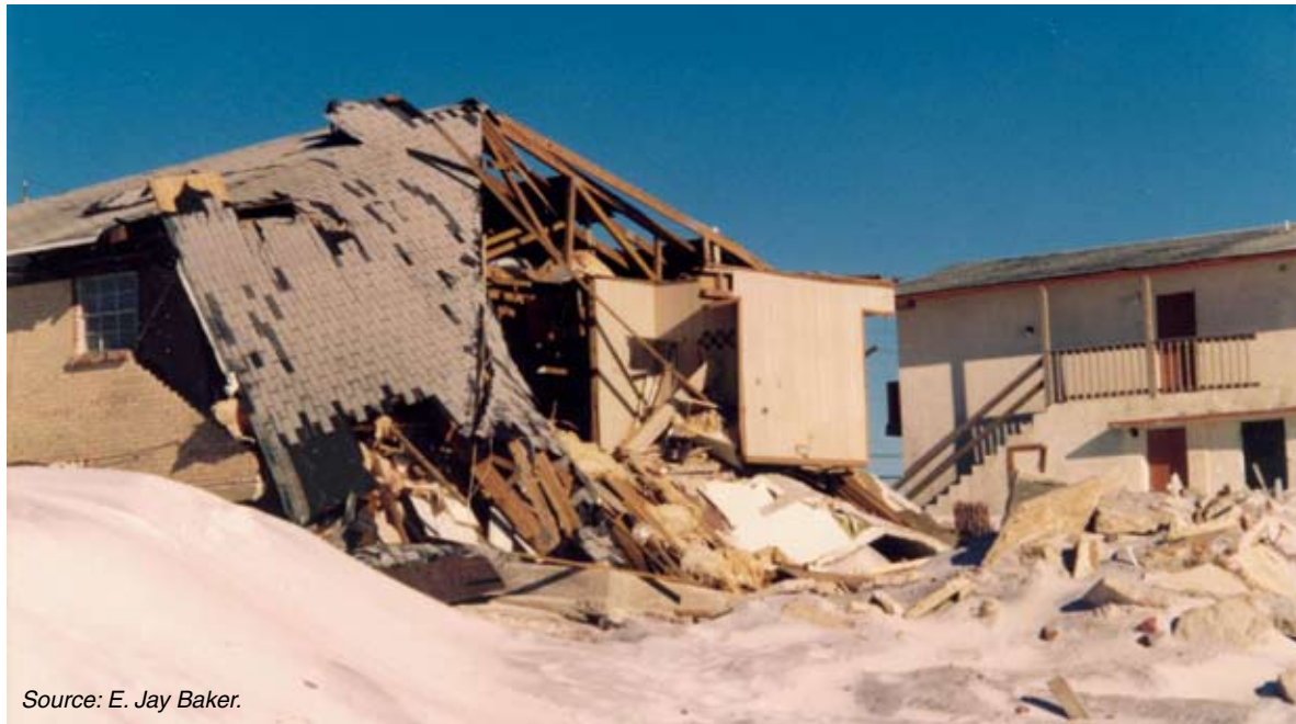
Figure 5.4: Storm surge damage from Hurricane Opal.
